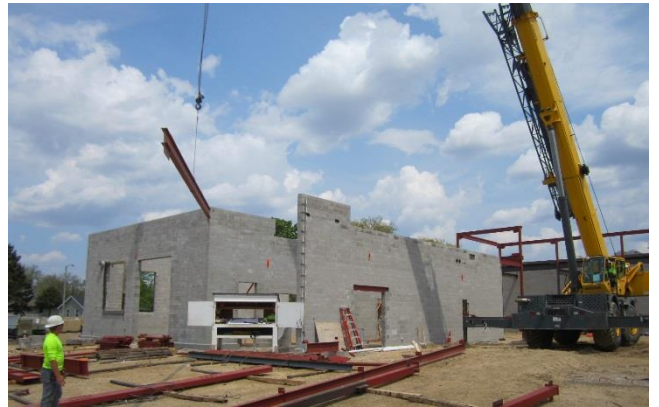
Structural steel is erected – in this picture, the crane is picking a roof beam for the ironworkers to set
