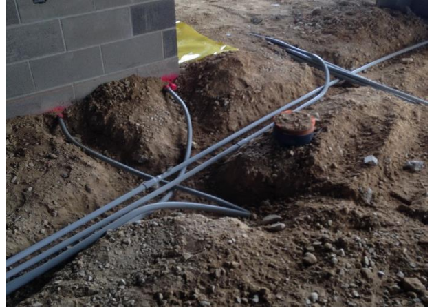
A network of underground conduit will provide power in the new addition.
