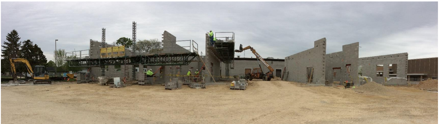
Load bearing masonry walls are completed and ready for steel erection. The masons are now working on the west exterior (non-bearing) walls. Structural steel will be delivered and erected starting next week!
