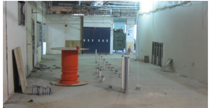
The existing concrete floors were cut open to allow new plumbing work to be installed underground before being backfilled and infilled with concrete. All of the pipes shown here will serve future bathroom fixtures
