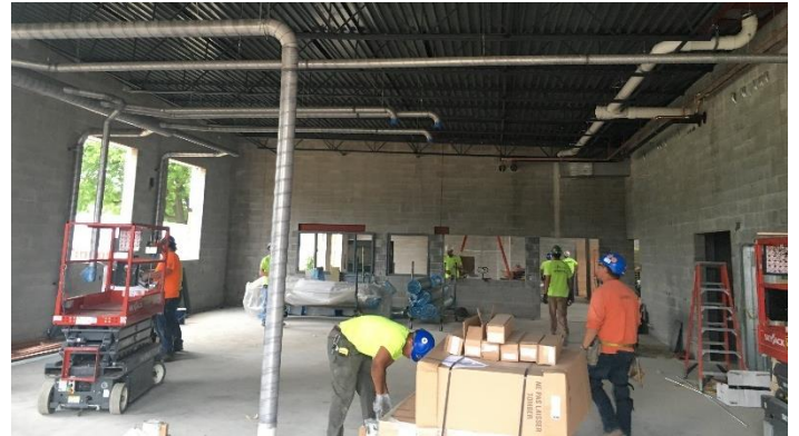
HVAC, plumbing and electrical crews are working to get ductwork, piping and conduit installed in preparation for painting
