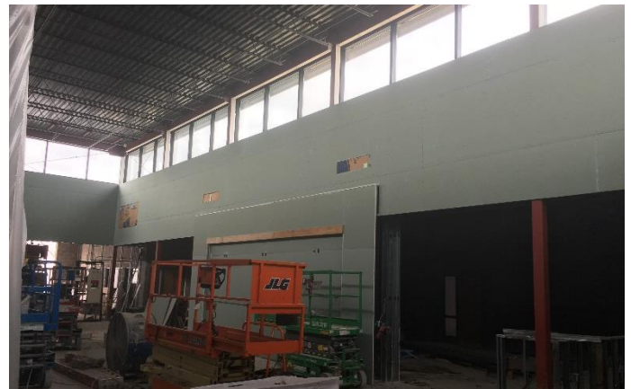
Drywall has been hung in the STEM collaboration space, and will be hung in the existing building starting next week
