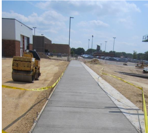
Concrete sidewalks have been poured, and the site is ready for asphalt paving.
