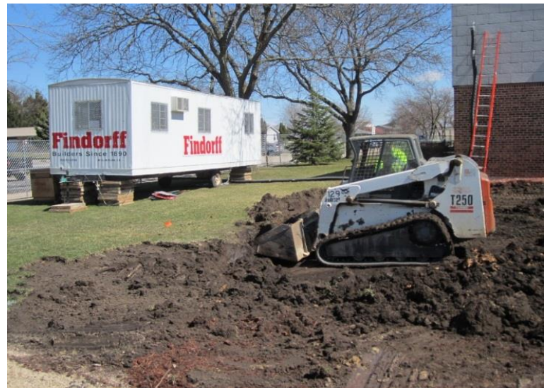
Site clearing has begun. Topsoil is being removed by the skid steer on the right. On the left is the Findorff job trailer which the Site Superintendent works out of.
