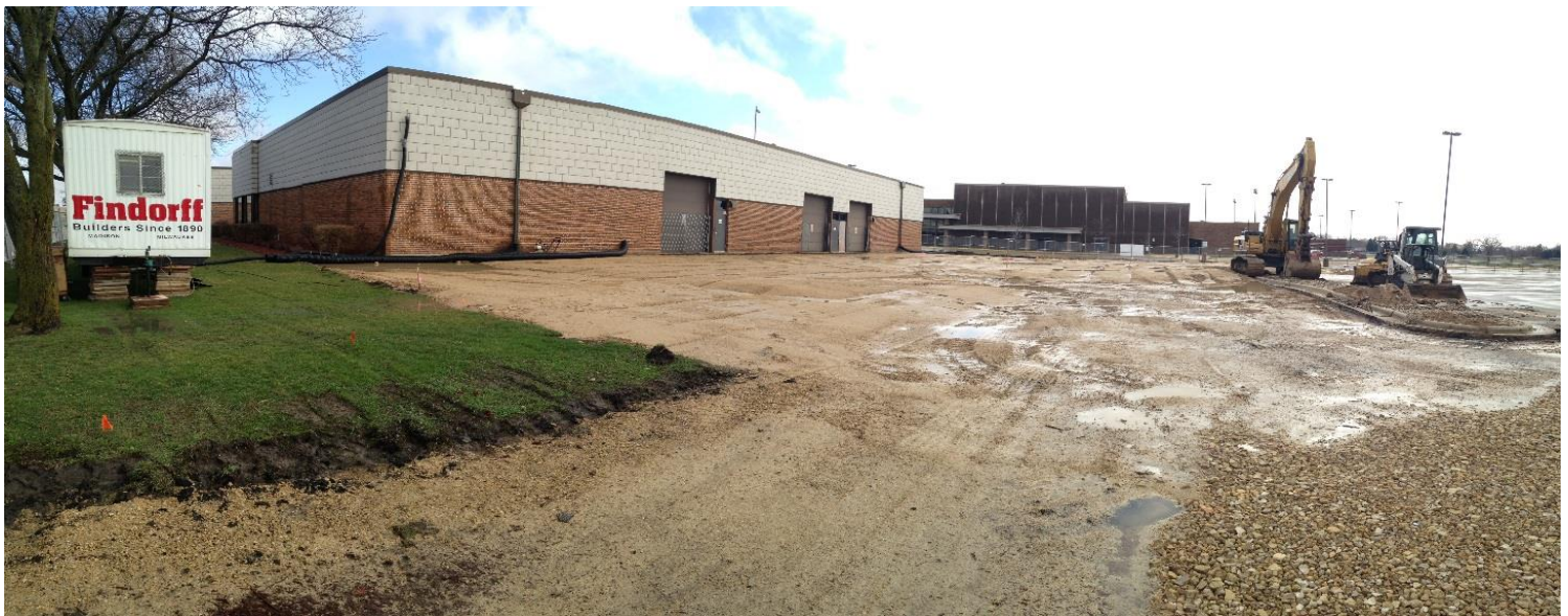
The building footprint has been prepared by removing the topsoil and adding the gravel sub base. Excavation equipment is staged on the right ready to begin digging!
