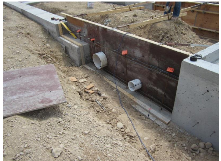
The stubs of piping in the wall have been installed to facilitate the future installation of underground plumbing work.
