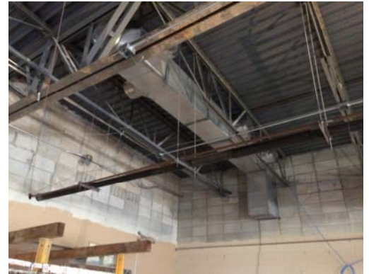
New duct work is installed for the new air handling unit that serves the remodeled STEM lab.
