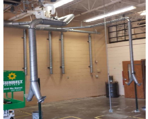
The new dust collection system is all roughed-in at the Middle School.
