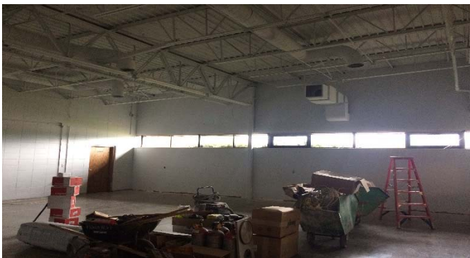
The STEM lab ceiling is painted as well as the walls. Ceiling grid will be installed next week.
