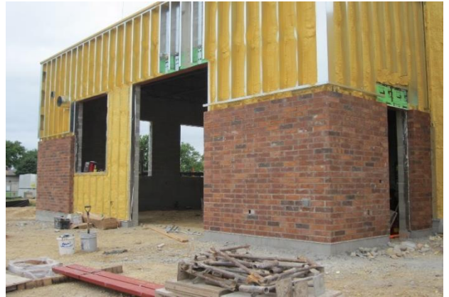
Brick veneer on the exterior of the addition, fiber cement panels on the upper walls will follow shortly
