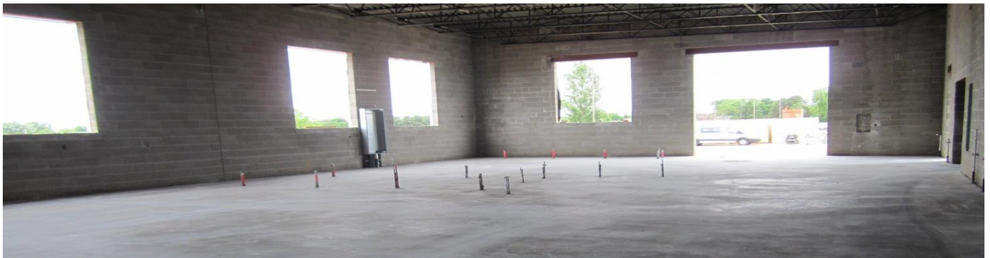
The cured concrete slab for the new metals lab shown above. The conduit stubs shown sticking from the slab will provide power to the welding booths.
