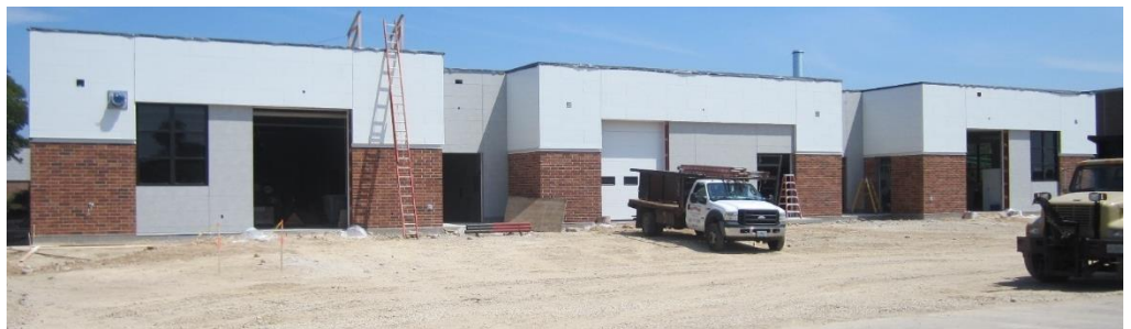
The exterior of the building is nearly complete – overhead doors have been installed, and "Nichiha" siding and exterior glazing are nearing completion! Site grading has begun in preparation for paving.
