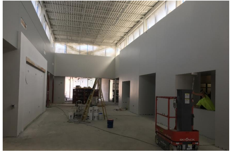
The new STEM space has been painted. Casework installation, MEP finishes, and ceiling installation will begin soon!
