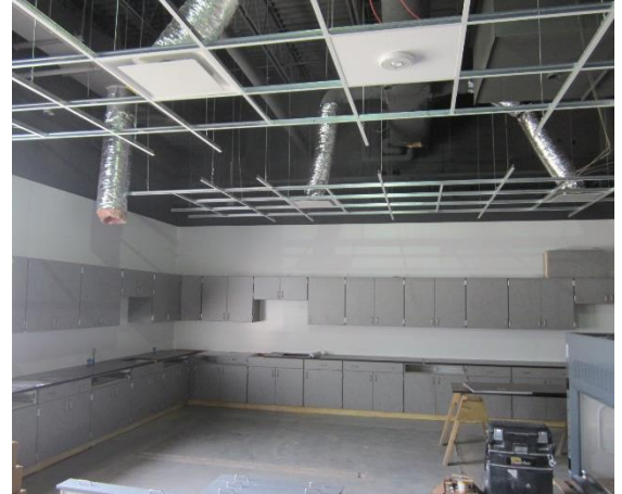
Casework has been installed in the science labs, along with ceiling grid. Epoxy countertops will be installed next!
