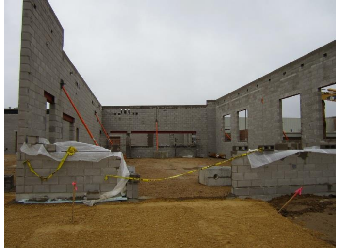
The south walls have been completed. The orange posts / braces stabilize the walls until the roof is installed.
