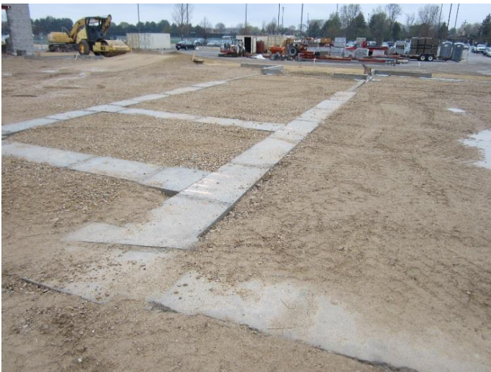
After the foundation walls are cured, insulation is placed and the wall has been backfill with soil the masons can begin on the walls.
